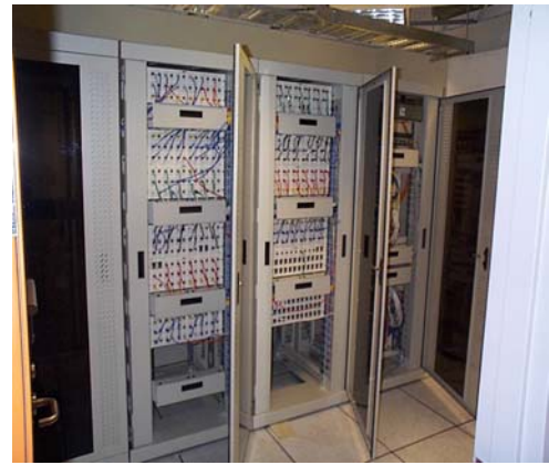
Infrastructure Engineered For Management & Performance
