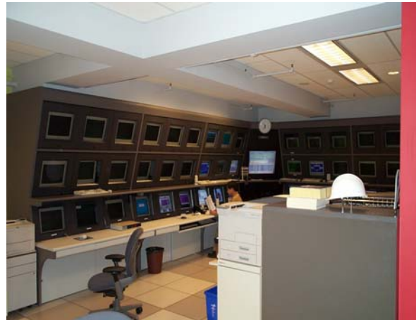
Recent Engineered Network Operation Centre (NOC)
