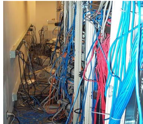
Disorganized Cable Jungle With High Exposure For Failure
