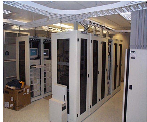
Engineered for High availability and fault tolerance
